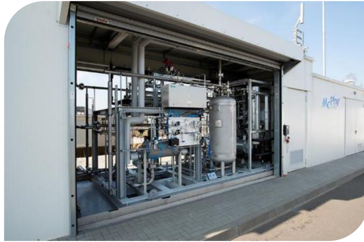
McLyzer 250 kg/day 42 bar system Electrolyzer
