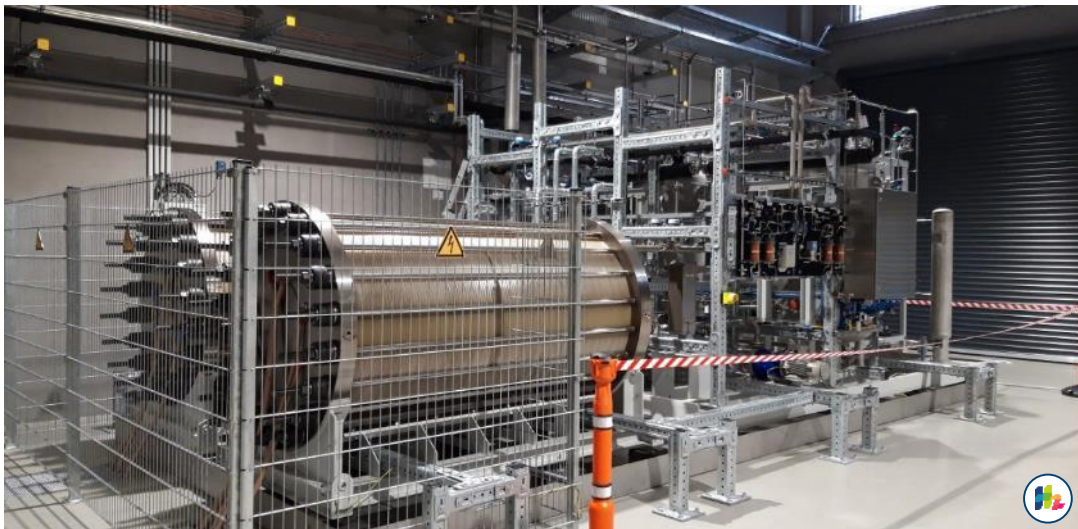
1 MW Electrolyzer (indoor installed)
