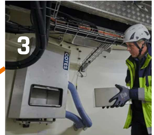
Wall mounted with ventilation
