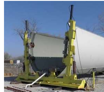
Assembly of a tower segment of the modular tubular steel tower (Modular tubular steel tower, 2014).
